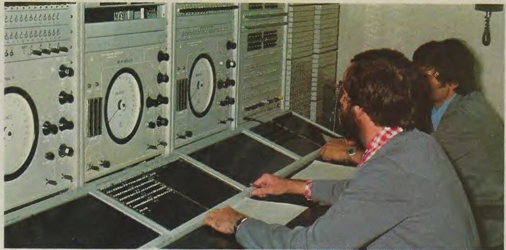
An overall view of the highly sophisticated monitoring panel in a modern 10C exchange.
