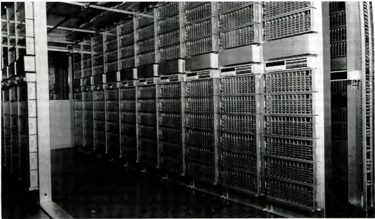
Fig. 5.1 — Crossbar Switch Racks
