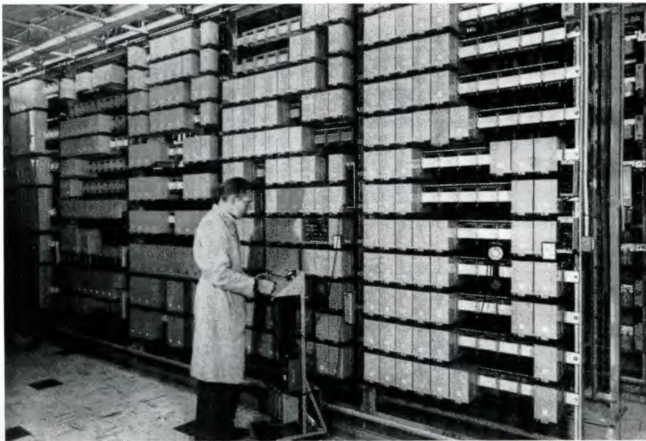
Fig. 3.1 — 2000 Type Equipment racks
