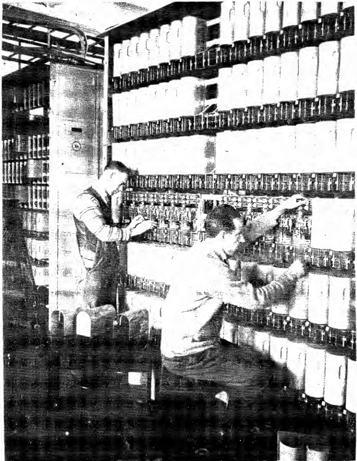
TECHNICIANS MAKING FINAL ADJUSTMENTS TO SELECTORS IN AN AUTOMATIC EXCHANGE PRIOR TO THE "CUT-OVER".
